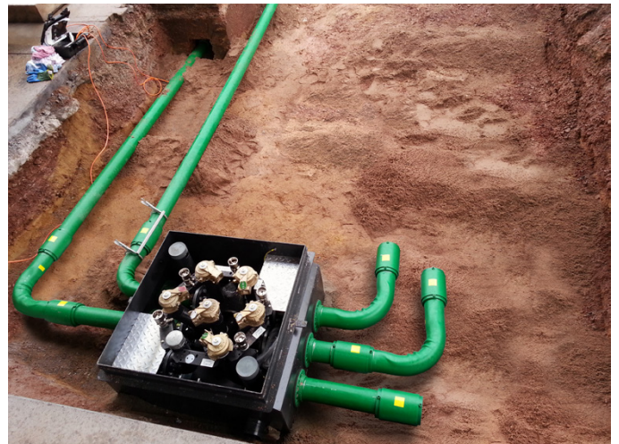
Once the plastic KPS piping was in position, the old steel piping was disconnected and the new KPS piping was connected
