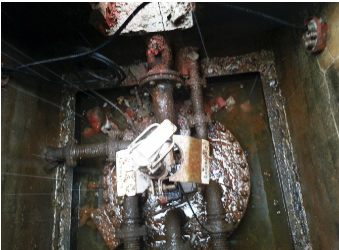
Previously installed steel piping had become damaged over time and started to rust
