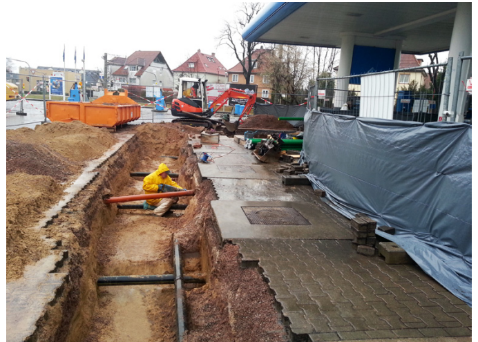
KPS piping was installed one level above the steel piping, preventing interruption of fuel sales
