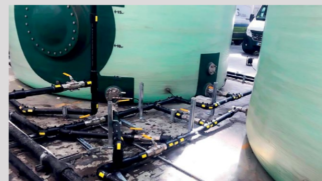
Maxol AdBlue Manufacturing Facility, Ireland
