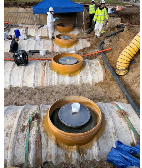
GRP chamber tank collars fibre-glassed to the GRP UST to retrofit the Fibrelite tank sumps
