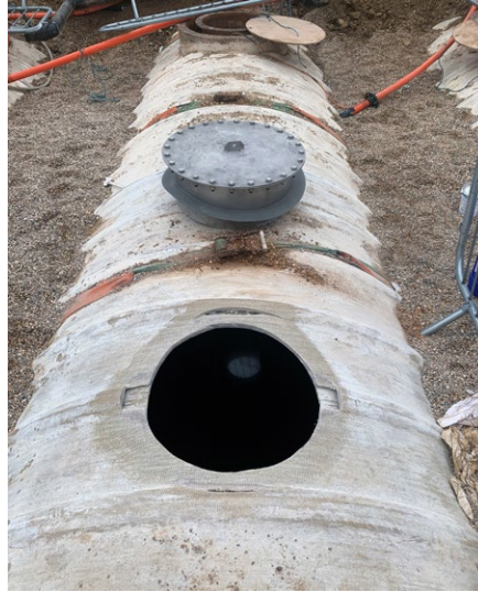
A solution which would interface with the existing GRP fuel tanks was required
