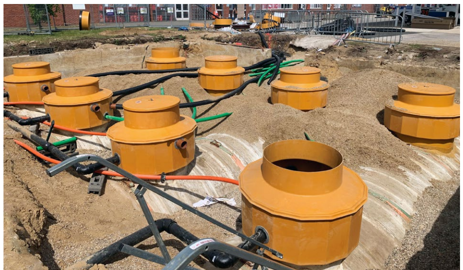
The Fibrelite and KPS technical team provided support from specification to installation
