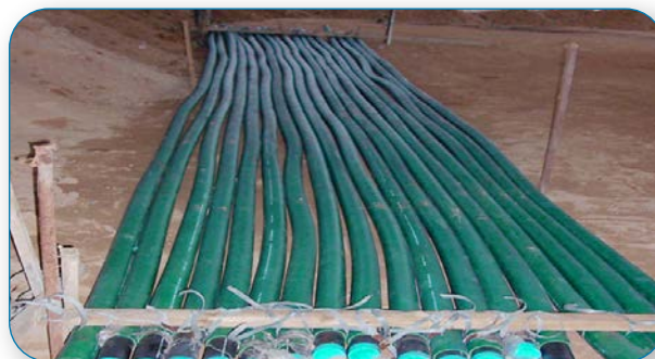
Straightening of coils.
