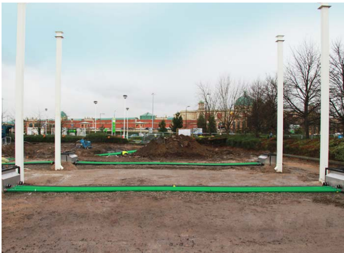
Client had a distance of 10m between pump islands.
