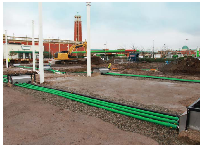
10m lengths of custom 75/63mm KPS straight pipe allowed fast installation without the need for a welding socket in middle.
