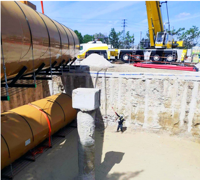
KPS conductive 4" pipe (125/110mm) was installed to connect the remote filling point to the fuel tanks
