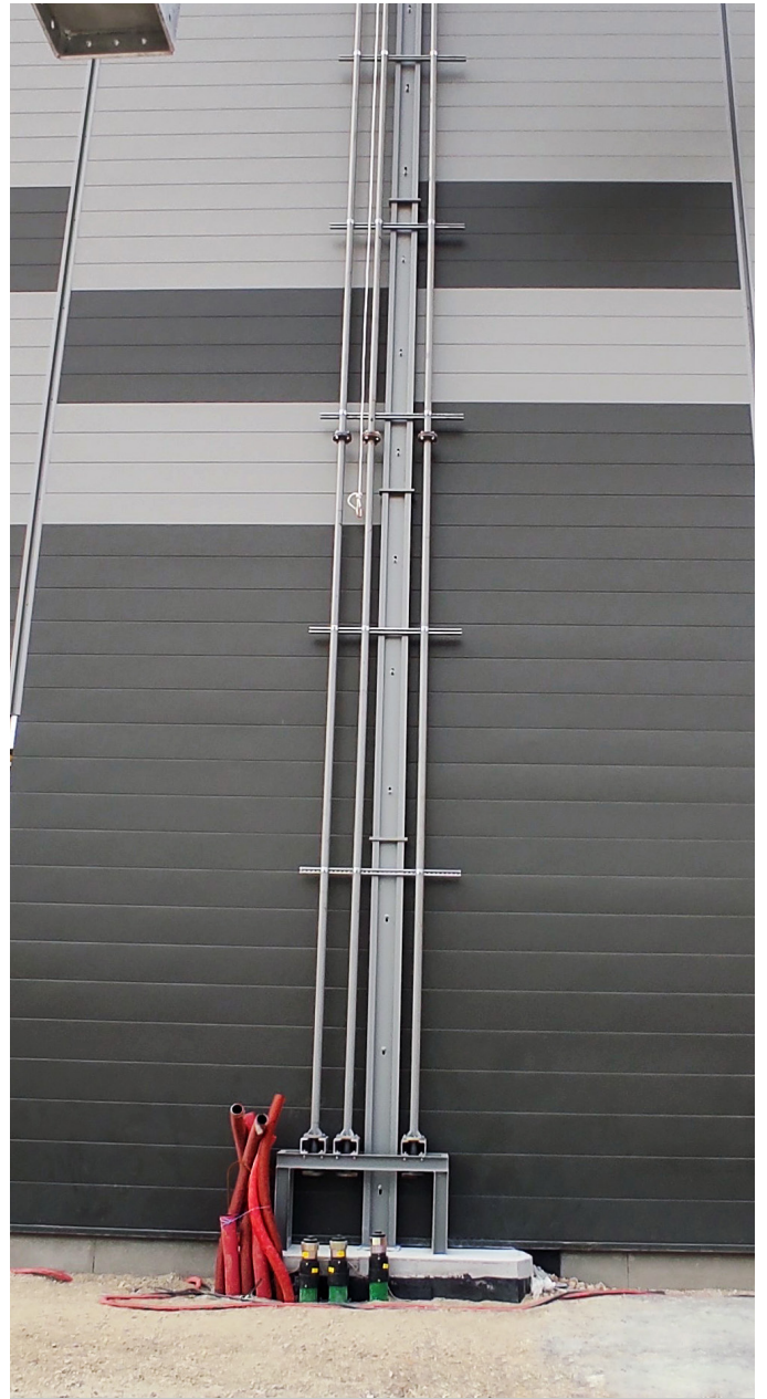
KPS' 2" (75/63mm) double wall piping was installed to connect fuel tanks to metal piping running up the outside wall of the facility
