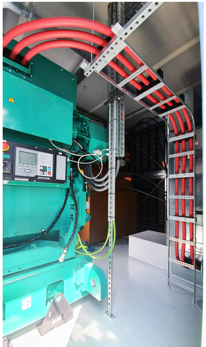
The diesel supply piping system connects below ground tanks to generators on the roof
