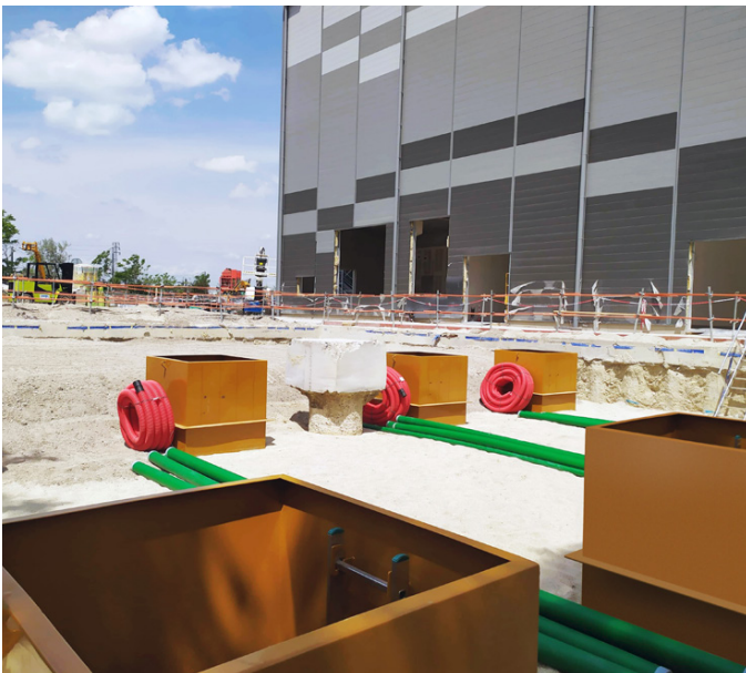
KPS 2" (75/63mm) conductive double wall piping connects fuel tanks to backup generators
