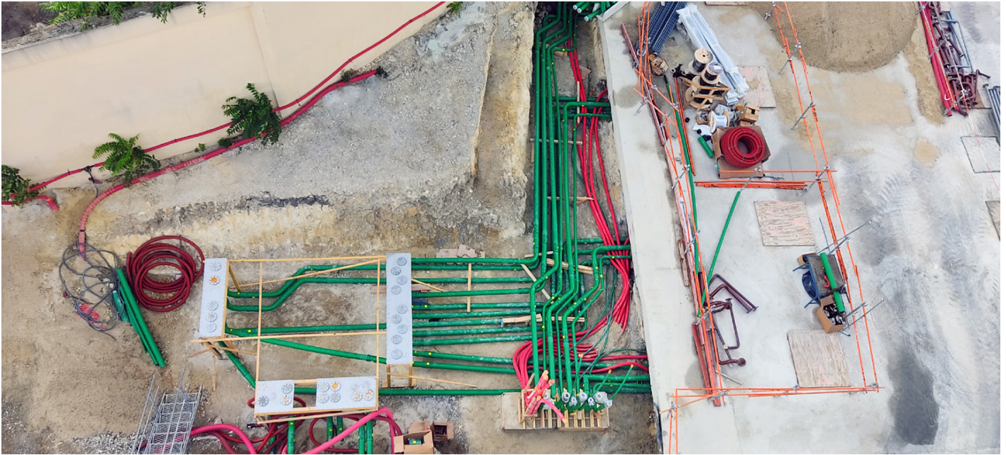
A new data centre facility in Paris, France specified KPS double wall piping to fuel backup generators
