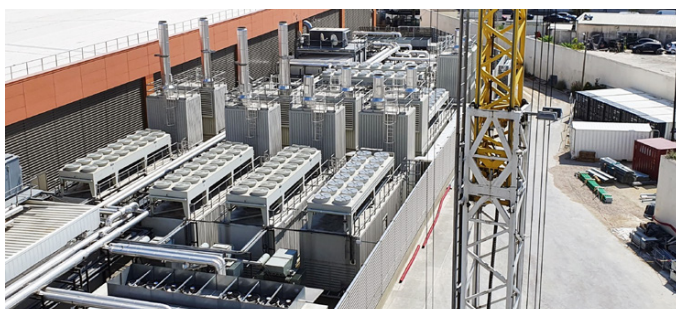
Data centre facilities require a number of backup generators to ensure an uninterrupted power supply
