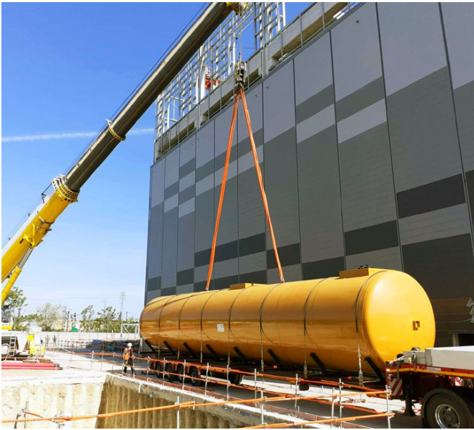
This facility required a high-performance piping system which would allow a 933 litre/minute flow rate
