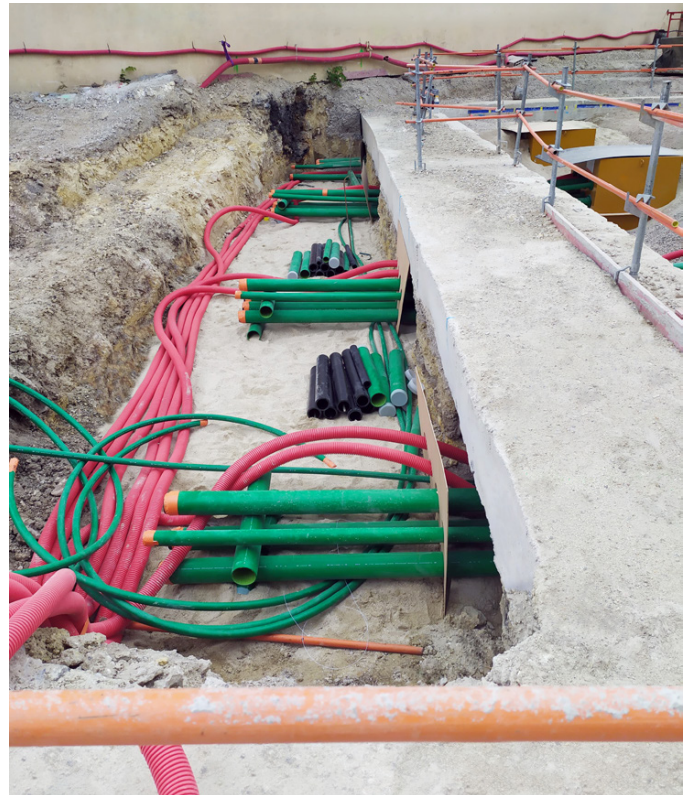
KPS piping is corrosion-free
