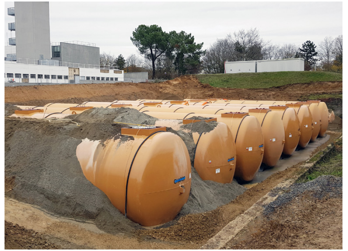
This project was a demanding district heating redevelopment project in Rennes, France
