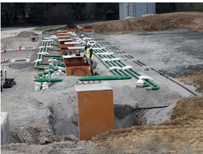
OPW provided a tailormade KPS piping solution
