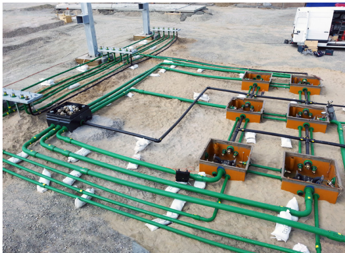
KPS piping had to be installed within 5 working days to meet the strict project deadline
