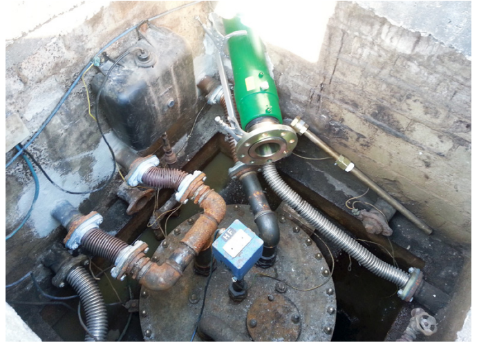
A hole was cut in the corner of each sump to allow the KPS termination fittings to enter
