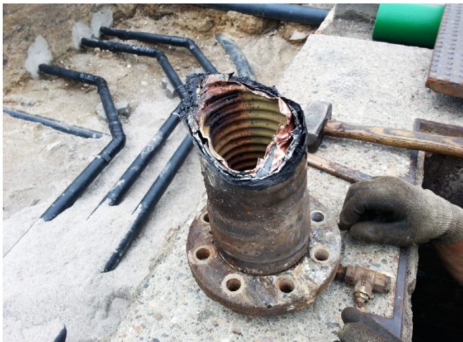
Previously installed corrugated steel and copper piping was damaged due to corrosion
