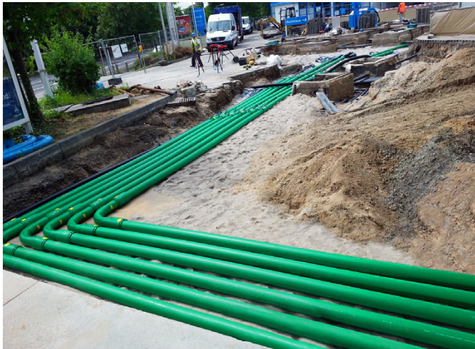
BP-Aral upgrades Leipzig site from steel to KPS plastic double wall piping
