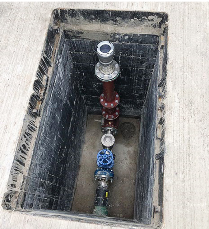
Complete below ground remote fill point
