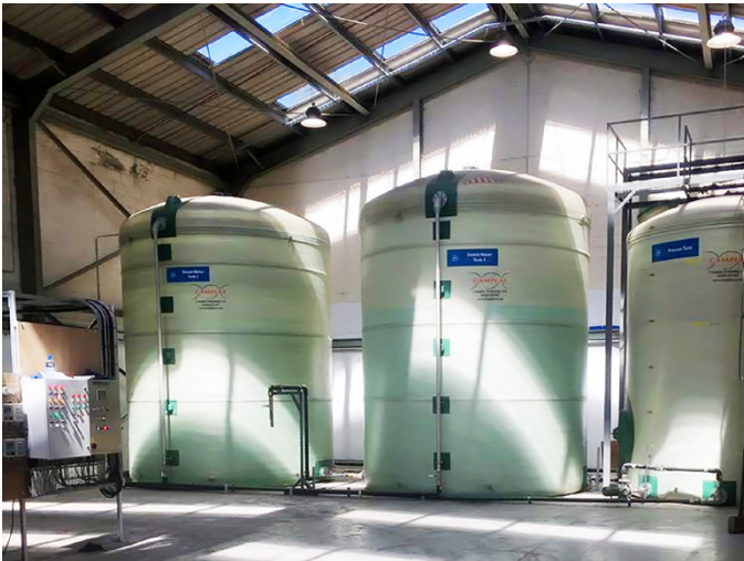
KPS piping proved the perfect solution for this new Maxol AdBlue production facility
