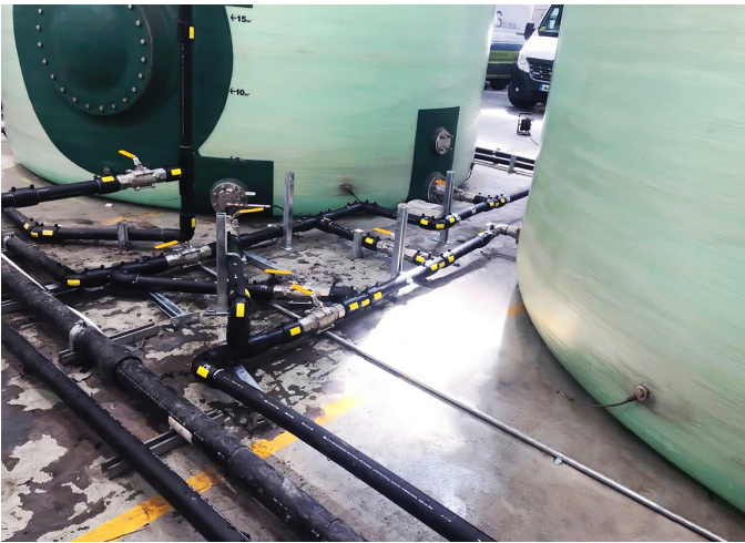
The KPS technical team worked with Petroleum Installations Solutions to create drawings using KPS' extensive range of fittings
