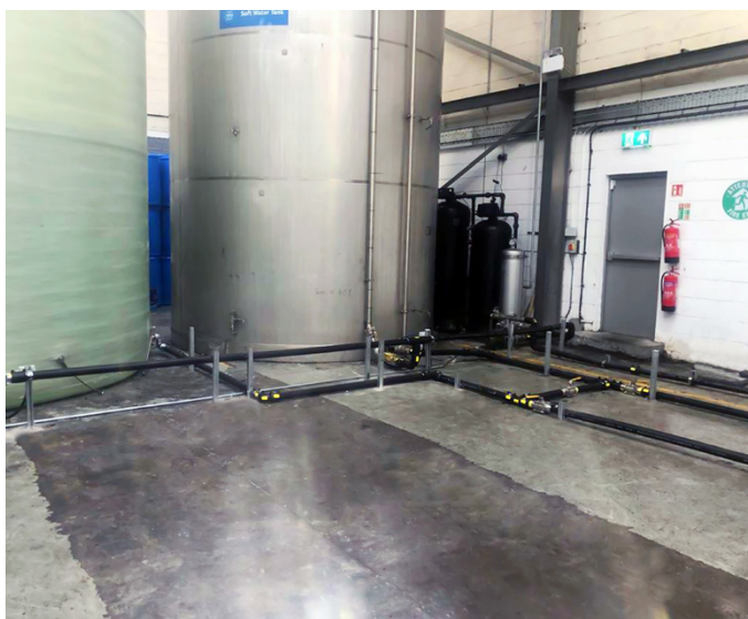
This project had a tight build schedule, so installation time was key
