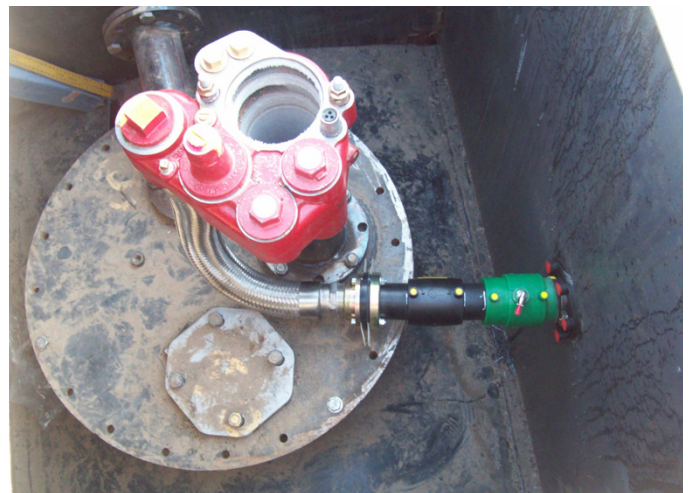
The KPS compact solution allowed for emergency valves to be installed under dispensers
