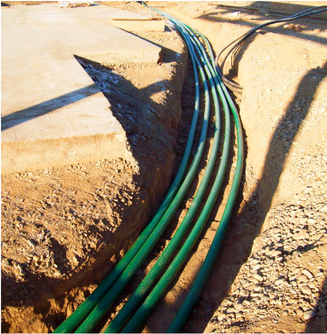
KPS provided long-term plastic piping system for pressure lines in Kazakhstan
