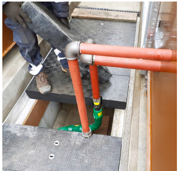
Apertures were required in some covers to accommodate pipework connecting from within the trench to above ground networks
