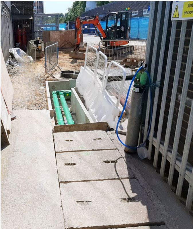
Previously existing concrete access covers were heavy and difficult to remove and replace
