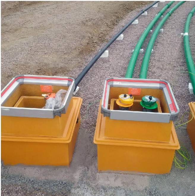
New sump and corbel utilised some items from existing product range to deliver a unique while cost effective solution
