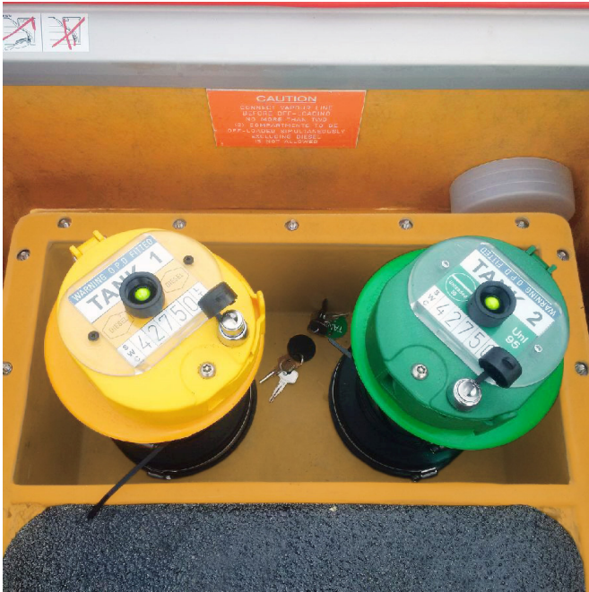
The fully conductive below ground remote fill systems are supplied with a non-slip working platform for the tanker driver to stand on
