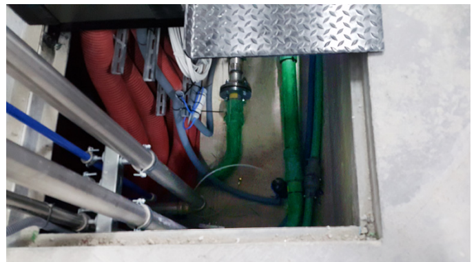
KPS piping allows the 933 litre/minute fuel flow rate required to supply diesel to the bus fleet
