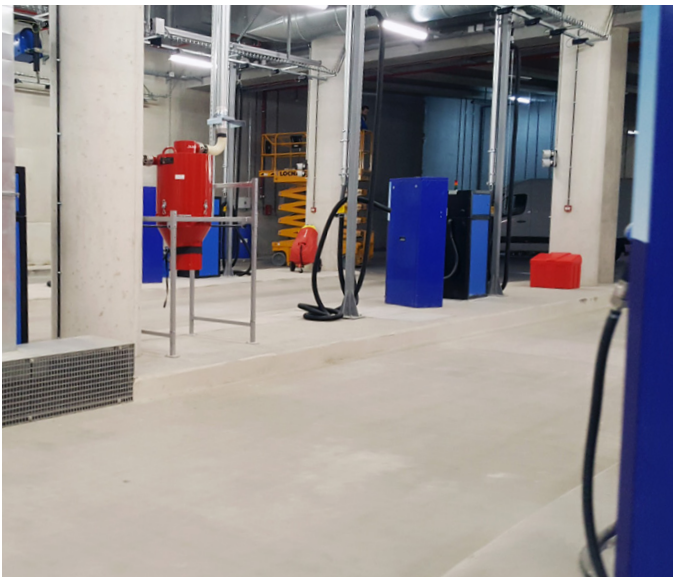
As the filling points were installed inside a garage building, a leak free zero permeation system was essential
