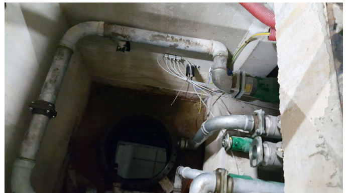
An interstitial space between the inner and outer pipes allows operators to monitor with the KPS leak detection system
