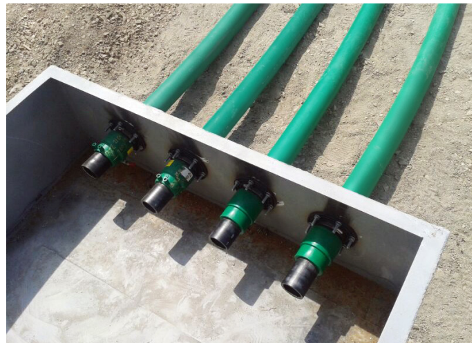
Training enabled a confident quality installation
