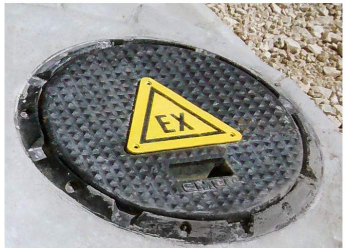
Previously used cast iron spill chamber
