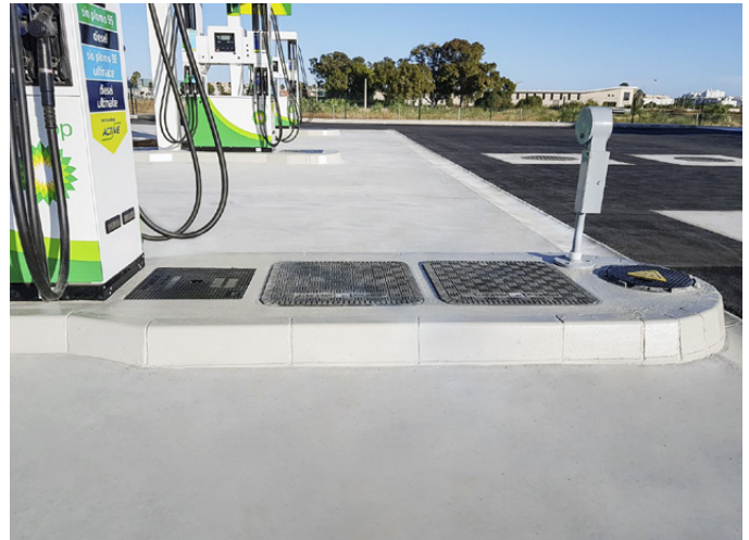
A full range of Fibrelite and KPS products was used to simplify supply and ensure quality
